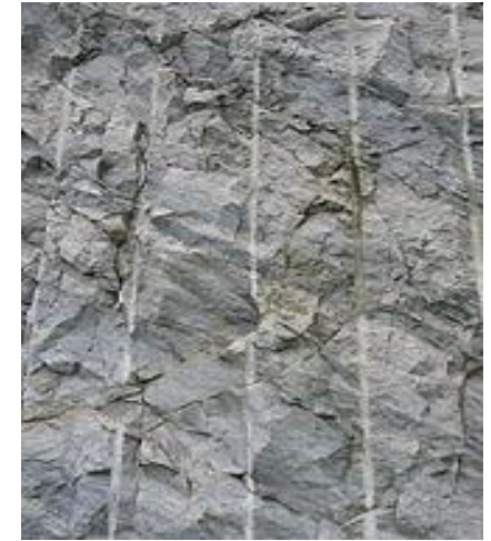
Rock surface newly blasted. This is called pre-split, it's a technique to leave a smooth face.
